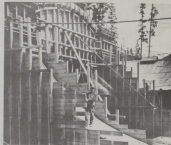
By early May 1927, the framing work for the concrete portal itself was in place (right) and after the concrete had been poured, example lettering was applied.
