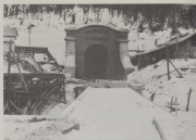
The West Portal awaits the track-laying crew on January 20, 1928, ten hours a month before the first train. (Moffat Tunnel Commission)
