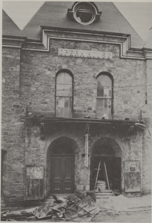
The Opera House during the initial stages of cleaning and restoration in 1932. An unidentified worker may be seen framed in the circular attic ventilator.
