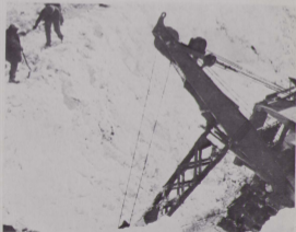
During the spring of 1930(?) the Needleton slide was so severe that it required the D&RGW ditcher, "Ox", to help clear the tracks.
