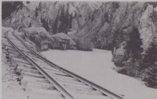
The tracks of the Silverton Northern, just north of the Silver Lake mill, were twisted when the flood of 1927 tore out the road bed. This same flood tore out the Silverton Northern bridge at the Silver Lake mill spur.
