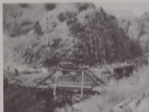
Old and new bridge construction are featured in this 1919 photograph documenting the building of the new "Carnegie" bridge between Gateway and Whitewater near Nine Mile Hill. (Photograph courtesy of Division of History, State Department of Highways, State of Colorado)
